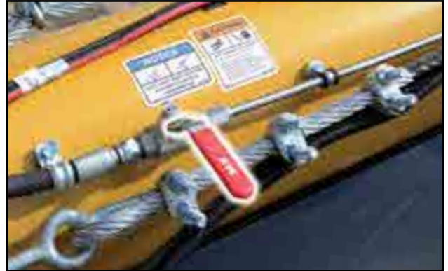
Fig 18 - Hydraulic valve to conveyor tube cylinders
